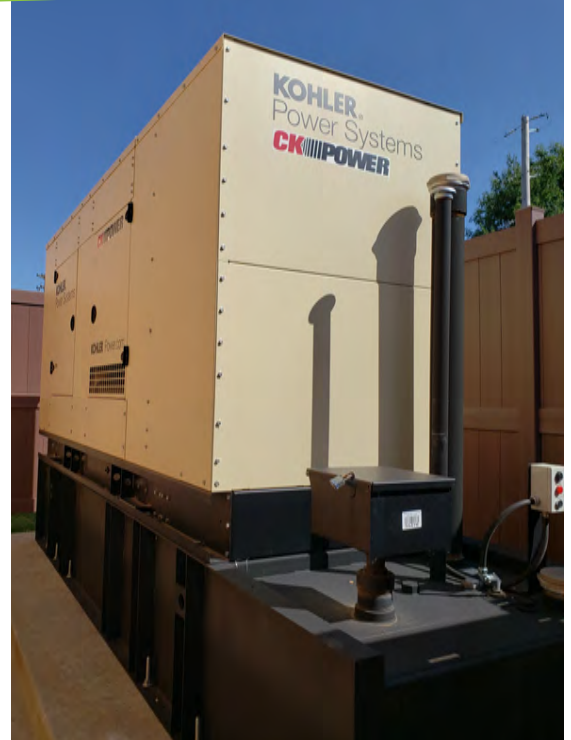
Surdex's Kohler 200Kw diesel-powered backup generator, which can generate electricity for four days on a single tank and be re-fueled indefinitely
